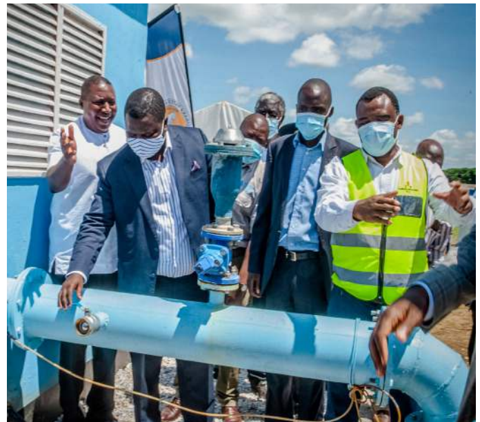
Installation of a 3.4 km pipeline to improve water access in a peri-urban community of 200,000 residents in Western Lusaka.
