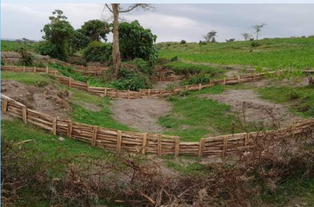
Erosion prevention structures set up in the Hawassa catchment under the Partnership.
