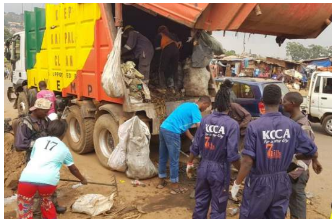
Community clean-up of drainage channels in cooperation with KCCA: The relationship between the City Authority and communities has improved through the partnership. © GIZ/Willy Ebong
